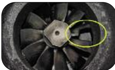
Figure 7 - Damaged Core Refund Hot wheel broken
