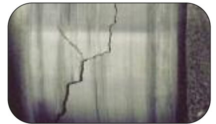
Figure 1 - No Core Refund Visible crack
