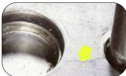
Figure 3 - Damaged Core Refund Top deck crack
